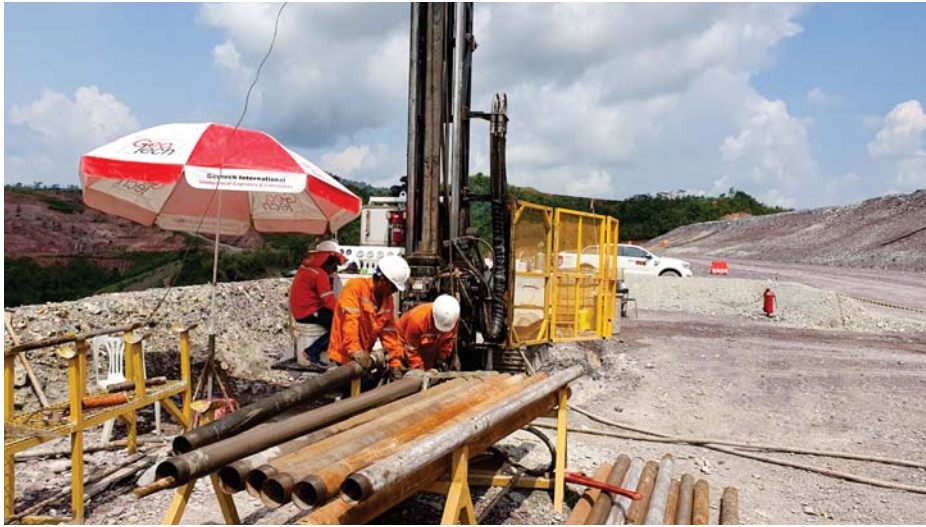
Geotech International performing geotechnical investigation and instrumentation installation at Phu Kham Mine tailings dam using Geotech International Boart Longyear drilling equipment - Lao PDR
